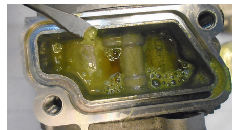
Jelly-like or crystallized sticky substance at the compressor's suction port. This severe pollution was caused by uncontrolled chemical reaction of moisture and additives like leak-stop agents. Only flushing can remove it all from the loop.
